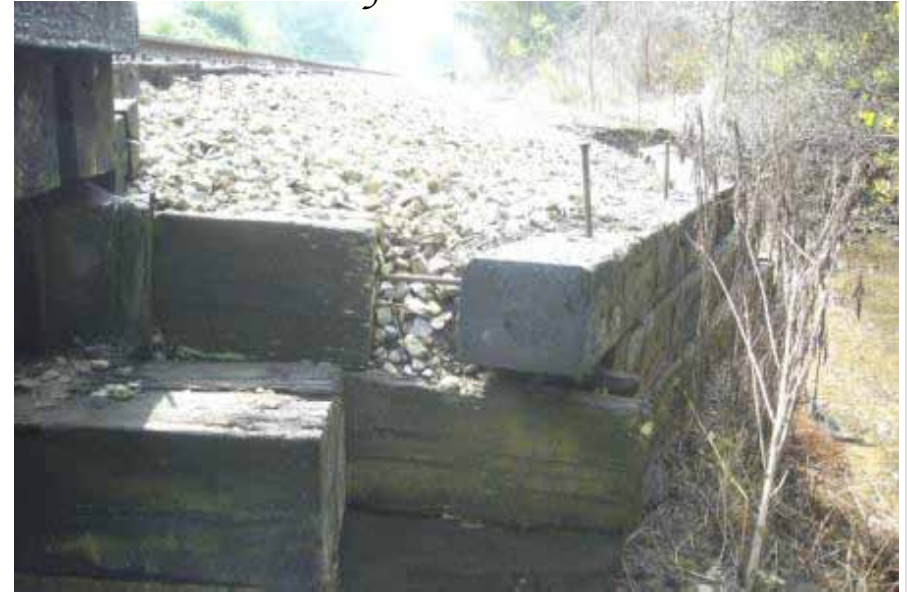
South Back Wall Deflection
