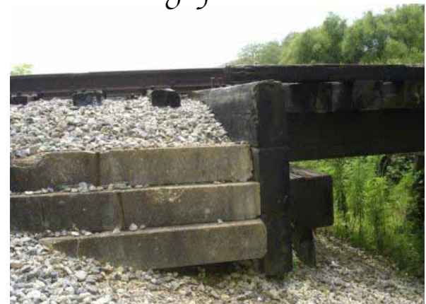
Undermining of South Back Wall
